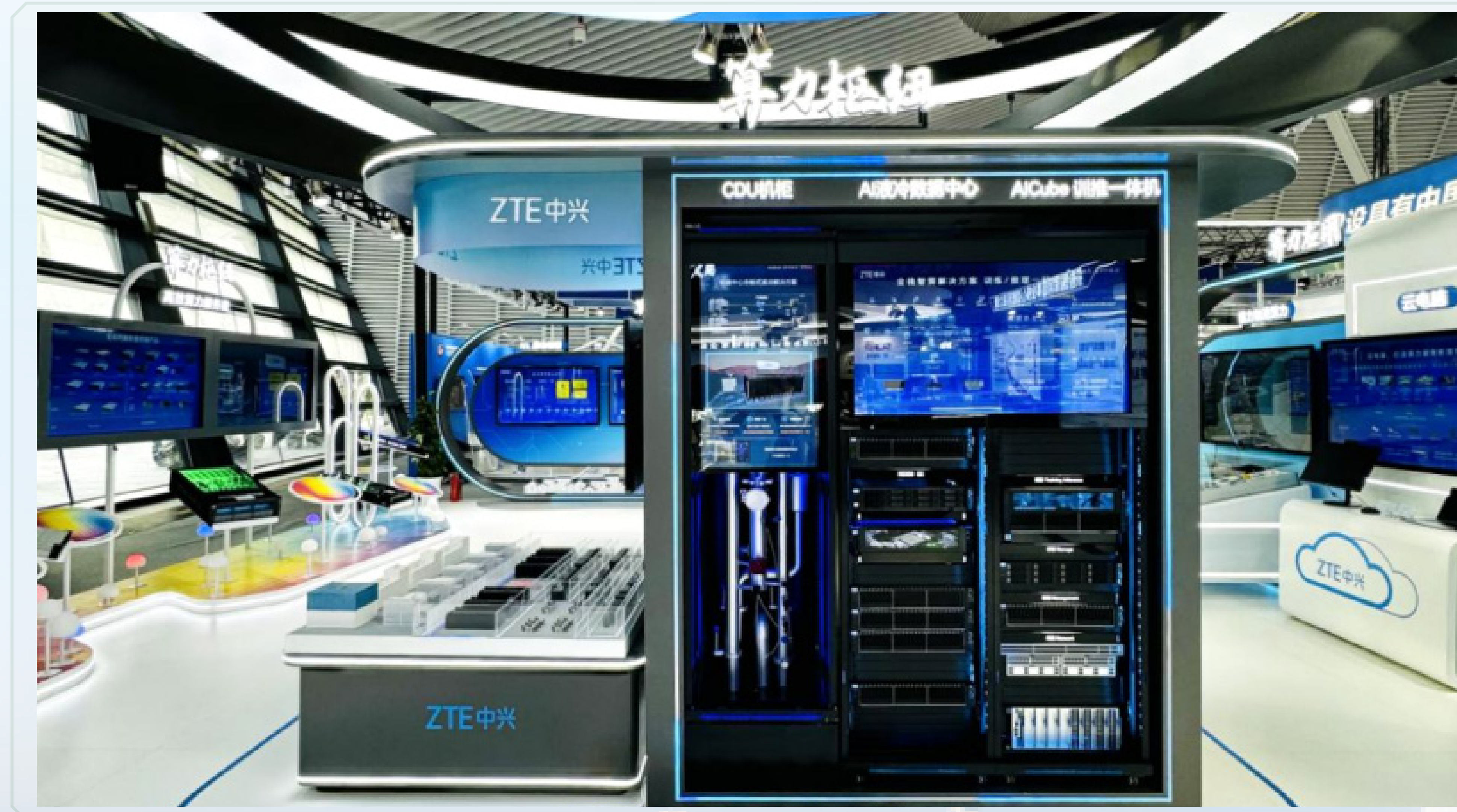
End-to-End Liquid-Cooled DC
