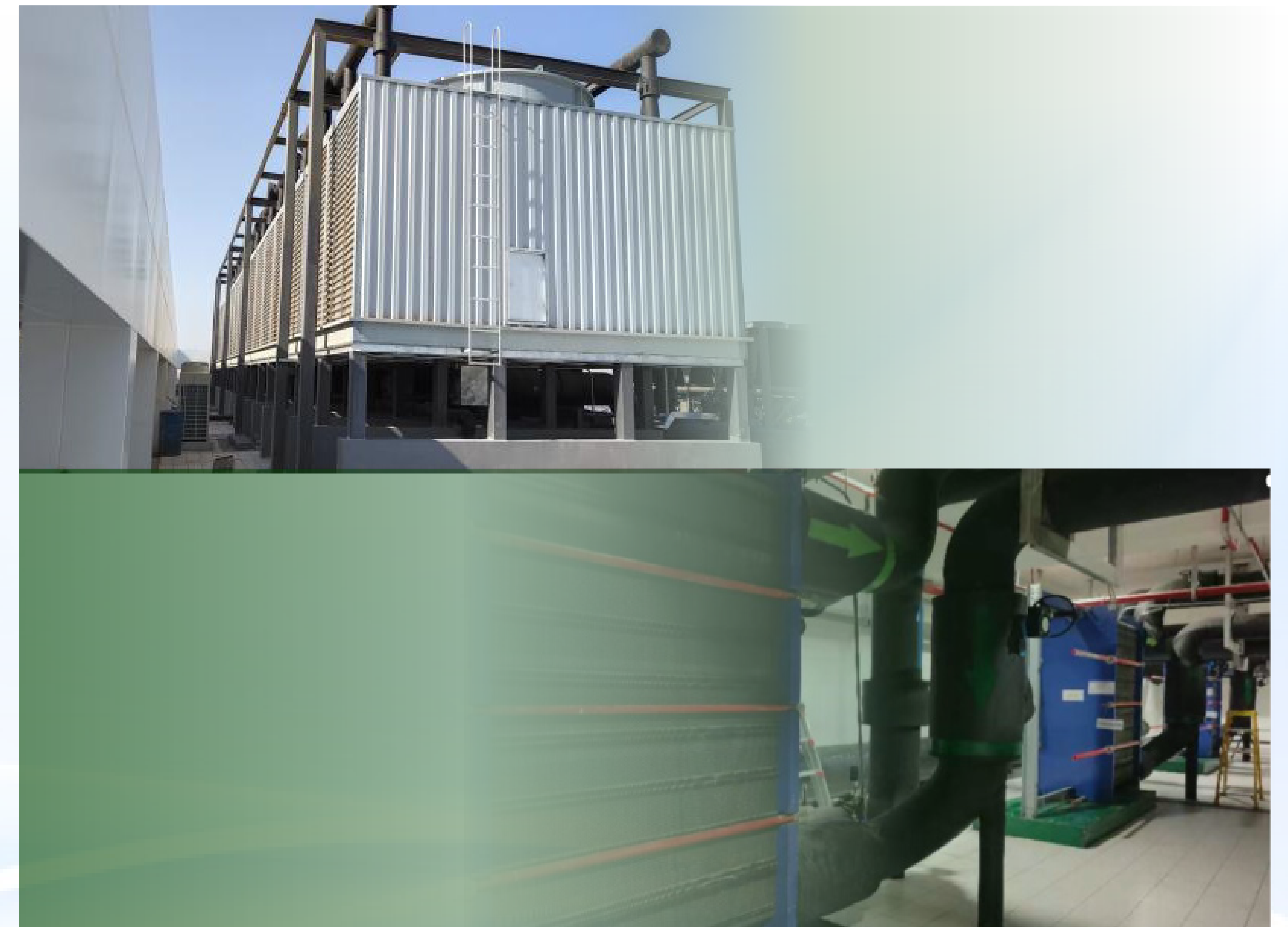
Cooling Tower and Plate Heat Exchangers that Use Natural Cooling Sources
